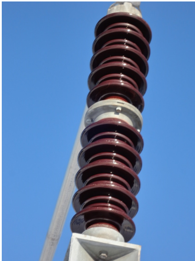
Figure 6: A multi-cone type insulator prone to failure due to cement growth
