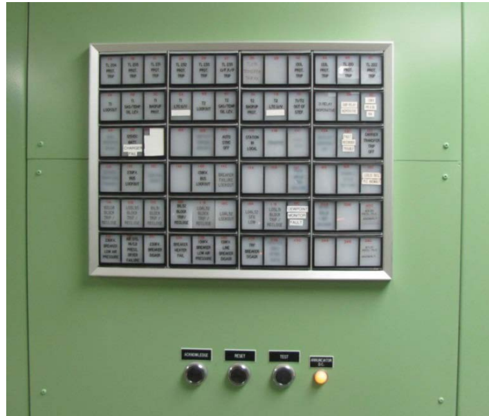
Figure 15: An annunciator commonly found in Hydro terminal stations
