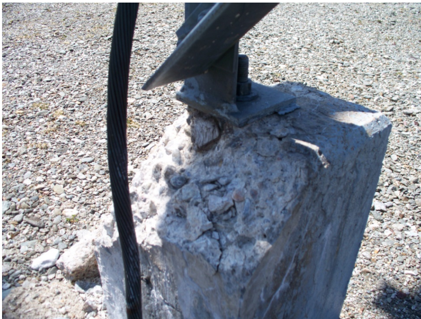
Figure 12: Structure B1T1 Bottom Brook Terminal Station
