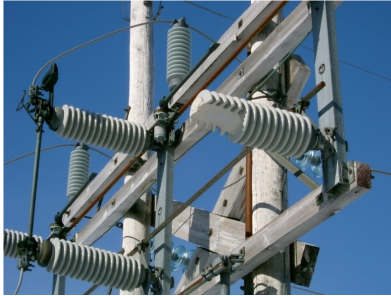
Figure 4: Broken insulator on 69 kV disconnect switch
