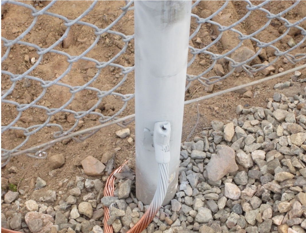
Figure 7: Typical grounding connection on terminal station fence
