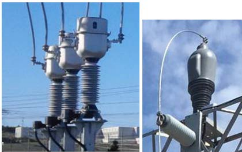
Figure 1: 69kV CT (Left) and PT (Right)
